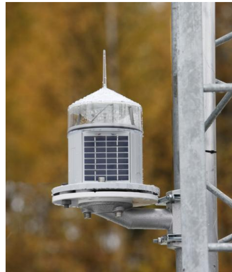
Picture 1 - SCA 110 installed in mast
